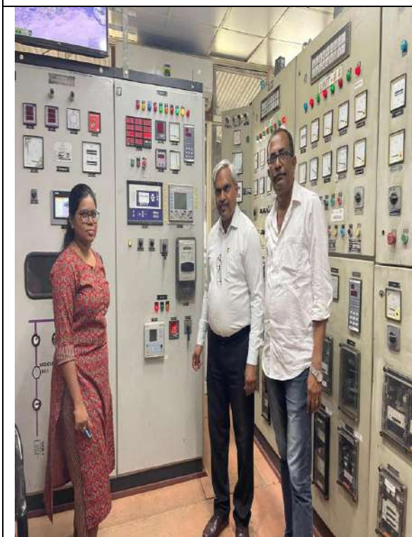
Electrical Control Panel
