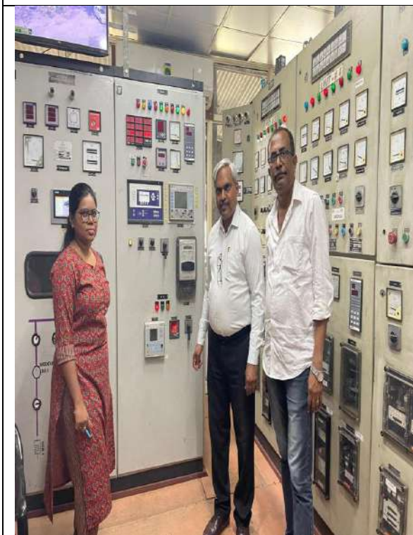
Electrical Control Panel
